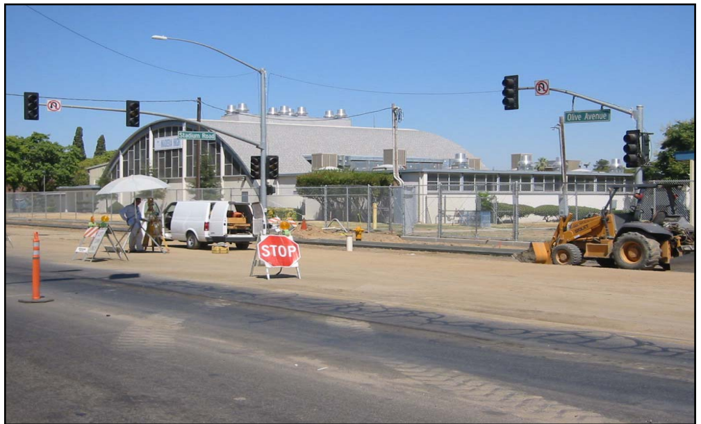
The Olive Avenue project is scheduled for completion by the end of October.
